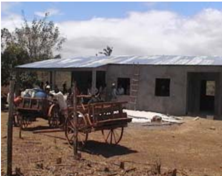
An oxcart brought water for the construction. In this very dry season barrels of water were hauled in to make cement.
